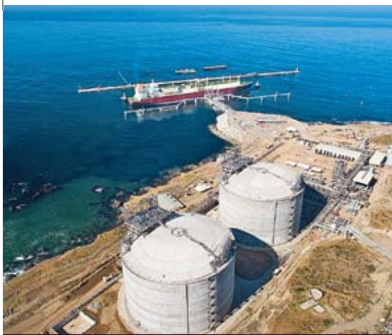
SEMPRA'S LNG RECEIPT TERMINAL ON THE BAJA CALIFORNIA PENINSULA RECEIVED ITS FIRST LNG SHIPMENT IN APRIL 2008.
